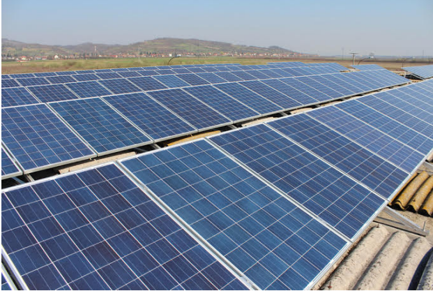
Upsolar and Upgrade Energy complete 653 kWp roof-mounted project in Croatia
